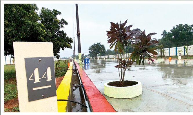
Well-Planned Storm Water Drainage & Street Lighting Facilities
